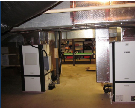
Two of six Bosch SM two-stage geothermal heat pumps installed in basement
