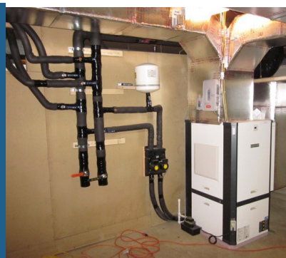
Geothermal flow system and manifold
